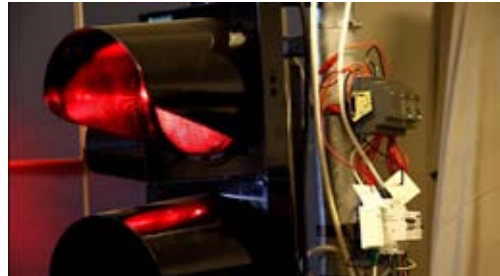
Public road traffic lights and control platform
